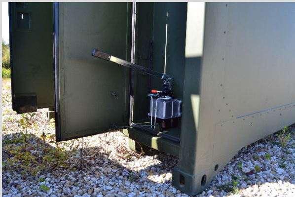
HYDRAULIC PUMP - SUPPORT ROLLERS
